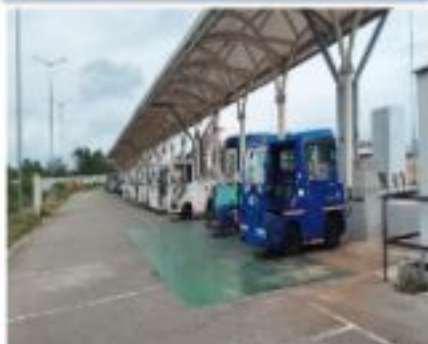
EV Charging Stations at Airside
