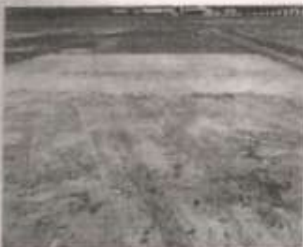
Photo 5. Abrasion on Repaired Patch
