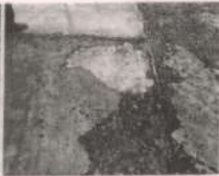
Photo 6. Delamination of Patched Material
