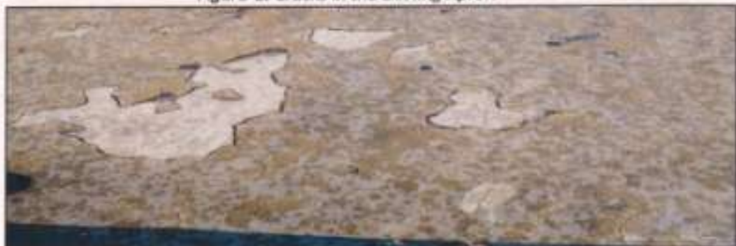
Figure 2: Cracks in the existing Apron
