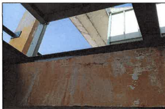
PH 05 - Severe cracks in RC members
