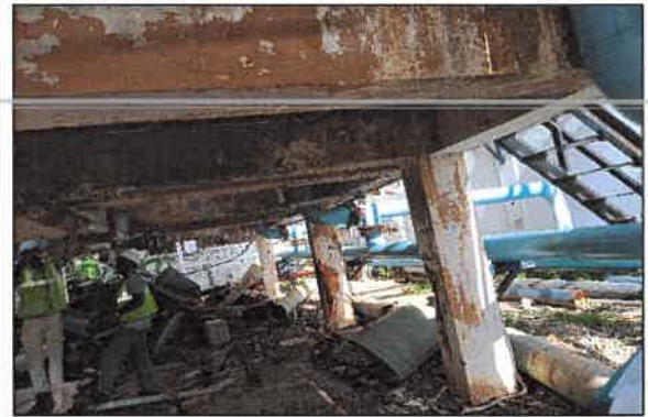
PH 04 - Dampness and damp patches in RC members
