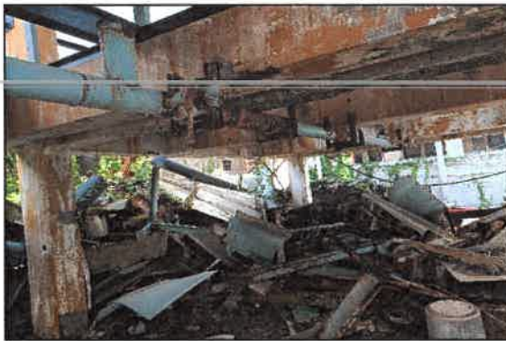
PH 03 - Dampness and damp patches in RC members
