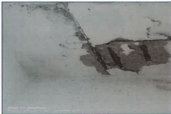
PH 07 - Cracks & exposure of corroded rebars in ceiling slab in internal side
